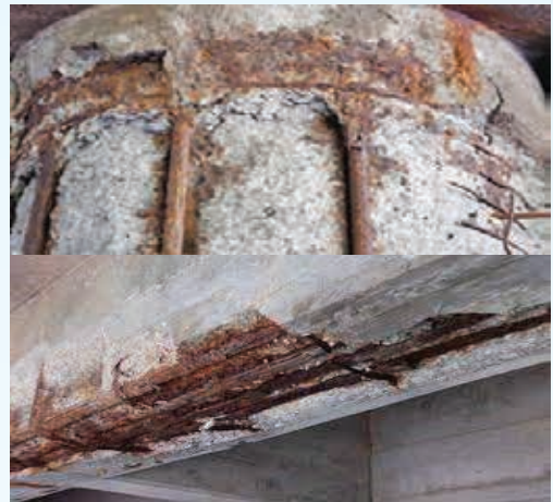
Concrete condition under harsh environment
